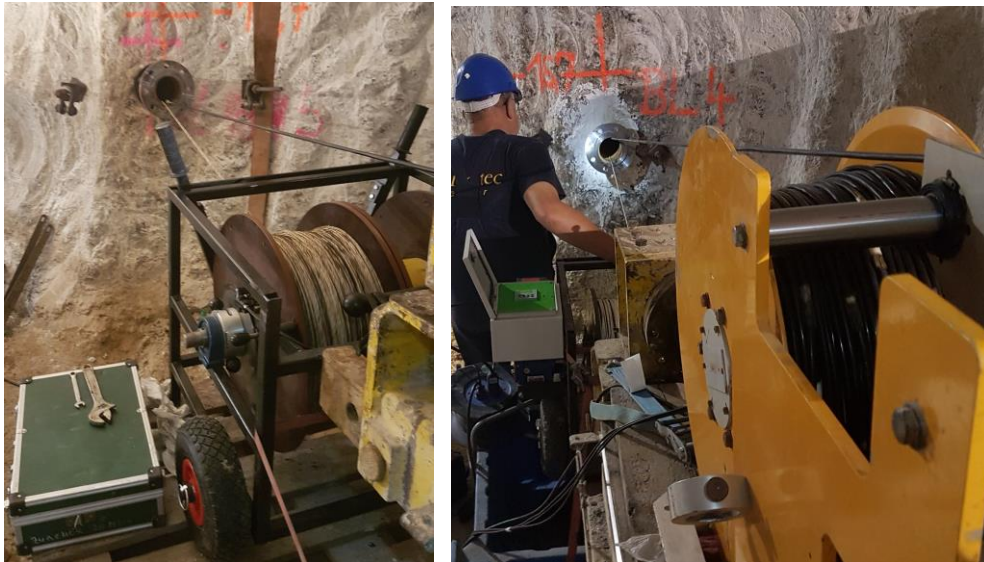
Fig. 4. Rope and cable winches to move the radar probes inside a deep horizontal borehole during measurement.
